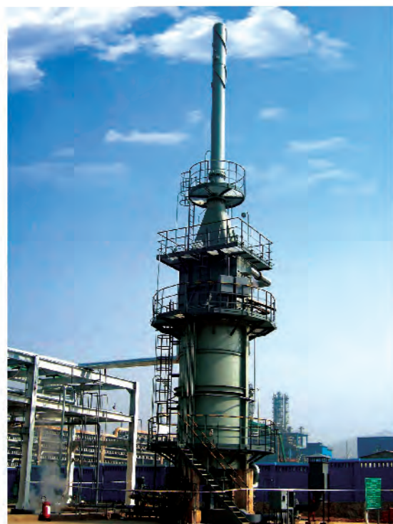
云南大为10万吨/年粗苯精制加热炉 Heater for 100,000 t/y crude benzol refining project of Yunnan Dawei
