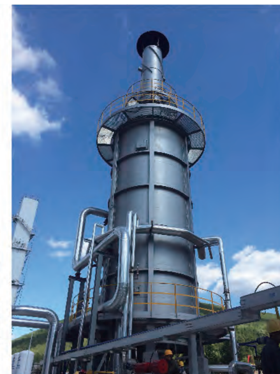
吉林通化合成氨项目加热炉 Heater for synthetic ammonia project of Jilin Tonghua Group
