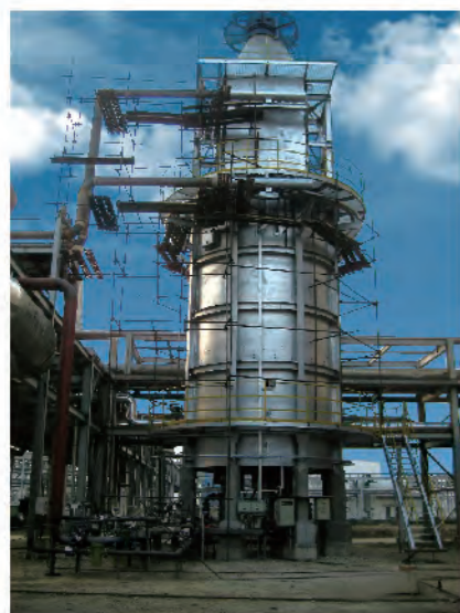
河南龙宇50万吨甲醇工程蒸汽过热炉 Heater for 500,000 t/y methanol plant of Henan Longyu Group
