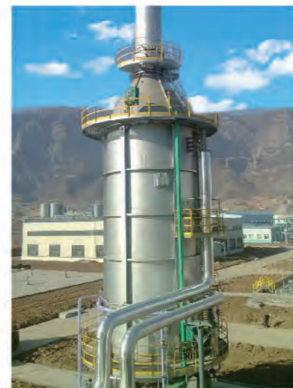
晋煤天庆合成氨项目加热炉 Heater for synthetic ammonia project of Jinmei Tianqing Group
