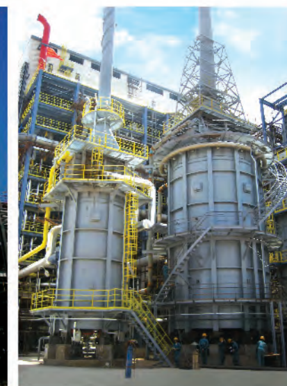
神华宁夏煤基烯烃项目再生气及氮气加热炉 Regeneration gas heater and nitrogen heater for coal-based olefin project of Shenhua Group
