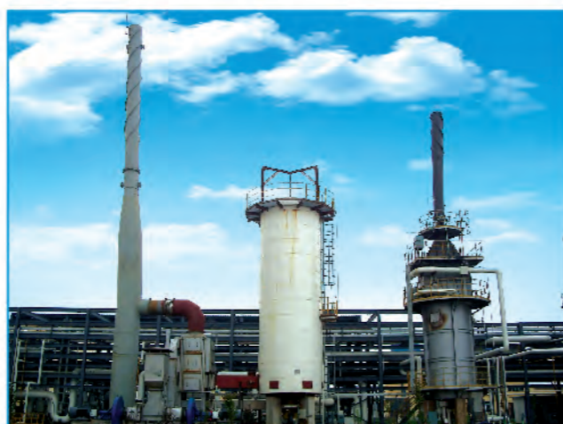
10万吨苯加氢装置导热油炉、加热炉 Hot oil heater and chemical heater for 100,000 tons benzene hydrogenation plant
