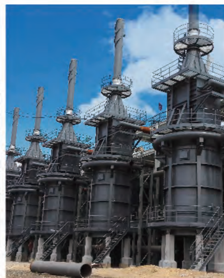
晋煤华昱100万吨甲醇清洁燃料再生气加热炉 Regeneration methanol clean fuel heating furnace for 1000,000 t/y of Jinmeihuayu Group
