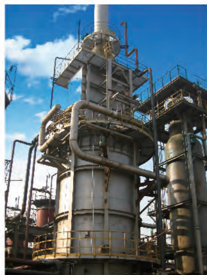
山东隆盛10万吨/年甲醇装置预热炉 Pre-heating furnace for 100,000 t/y methanol plant of Shandong Longsheng Group
