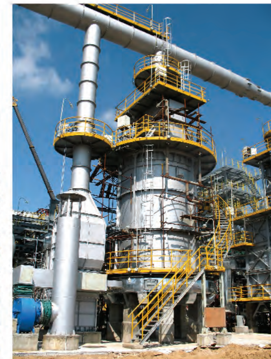
沥青改制项目加热炉 Heater for asphalt upgrading project
