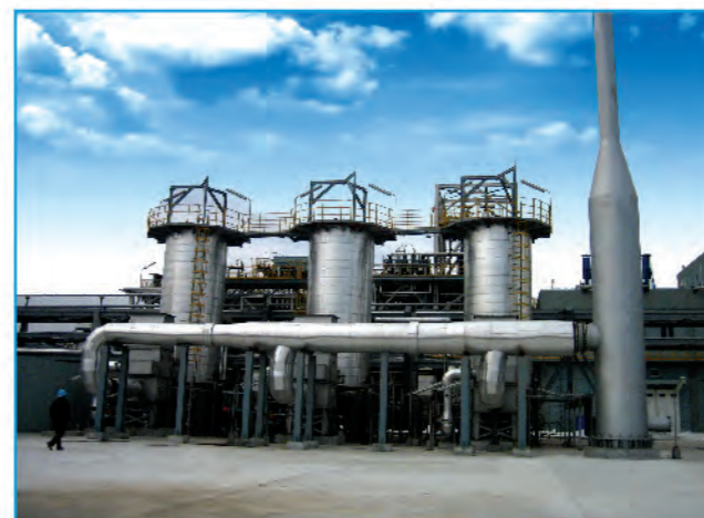
上海高桥分公司20万吨/年ABS装置 3X300万大卡/小时热媒站 3 sets of 3Mkcal/h hot oil heater station for 200,000 tons/y ABS plant of GaoQiao Petrochemical Corp., ShangHai Sinopec
