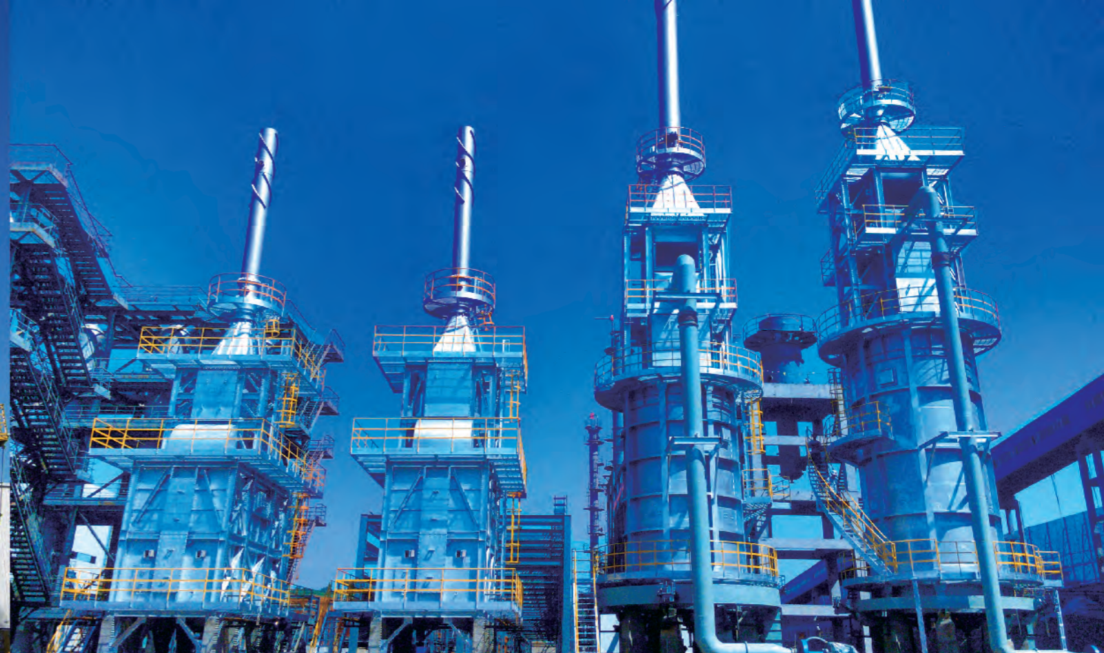
加热炉单元总包工程（山西南耀15万吨煤焦油加氢工程） Heater package EPC project (Shanxi Nanyao group 150000tons/y coal-to-oil Hydrogenation project)
