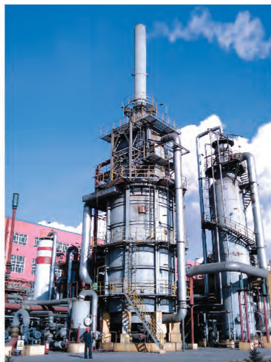
内蒙庆华20万吨/年甲醇装置预热炉 Pre-heating furnace for 200,000 t/y methanol plant of Inner Mongolia Qinghua Group
