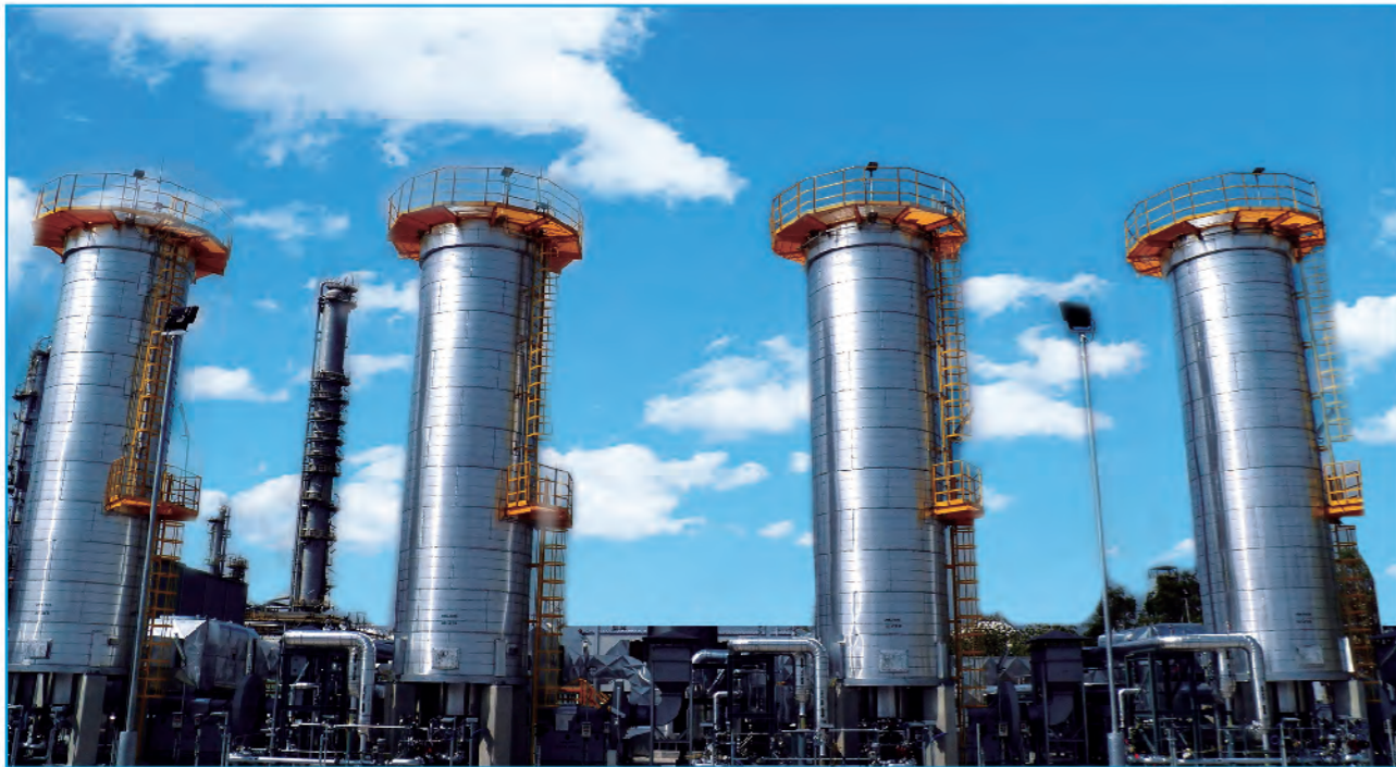
泰国PPT热媒站现场 Thailand PTT hot oil heater station
