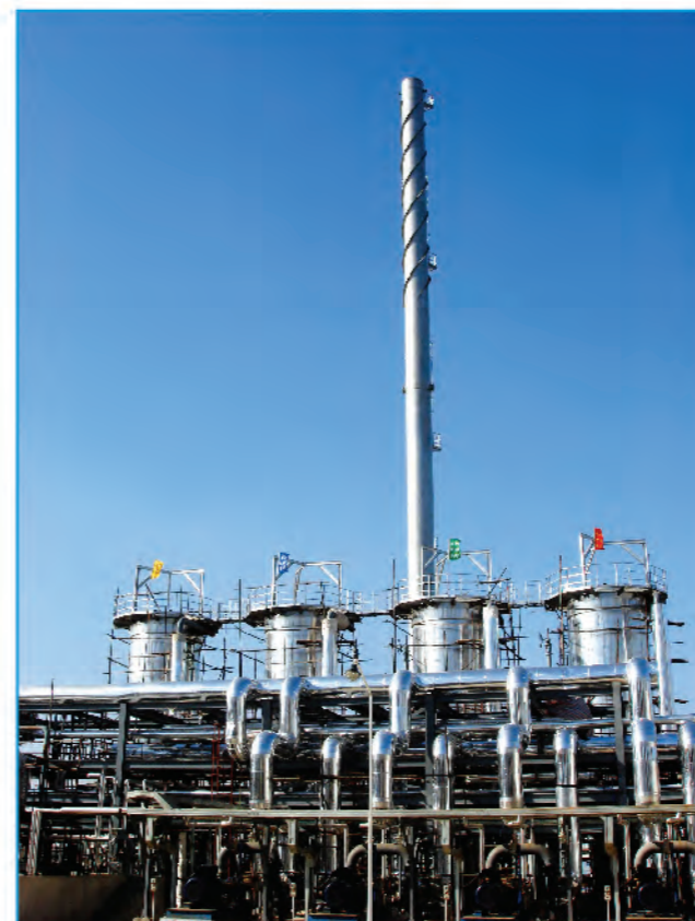
辽阳石化60万吨PTA装置4X1200万大卡/小时热媒站 4 sets of 12Mkcal/h hot oil heater station for 600,000 tons PTA plant of Liaoh Petrochemical Corp.
