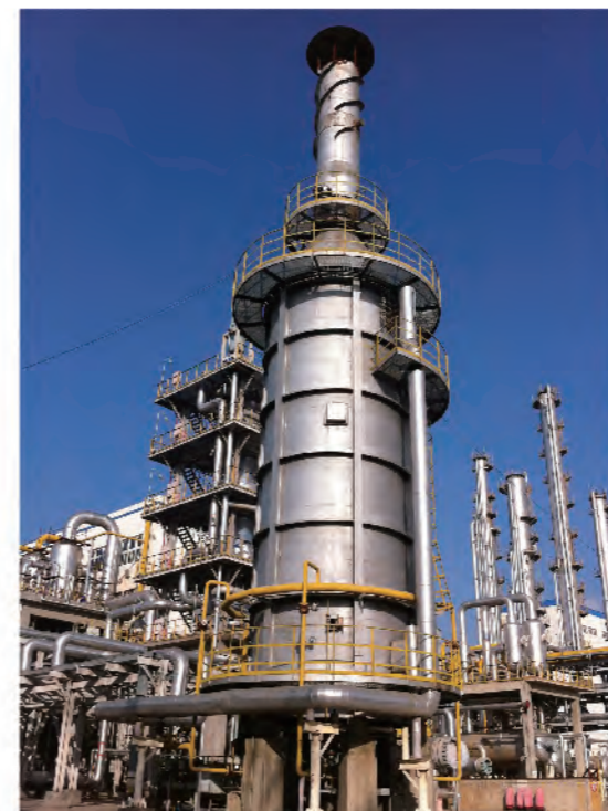
国电赤峰合成氨项目加热炉 Heater for synthetic ammonia project of Guodian Chifeng Group
