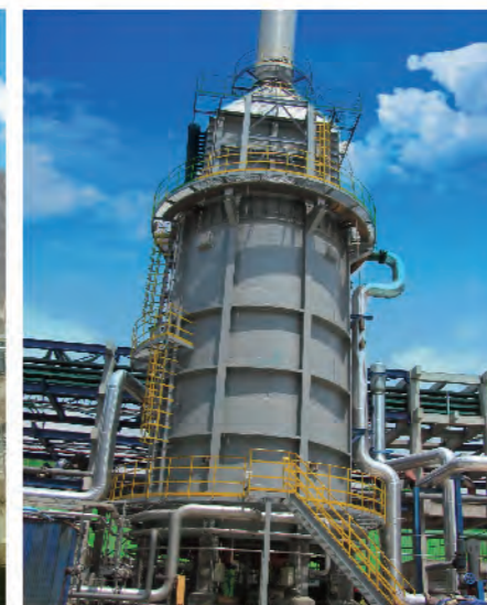
内蒙东华60万吨甲醇工程蒸汽过热炉 Heater for 600,000 t/y methanol plant of Inner Mongolia Donghua Group
