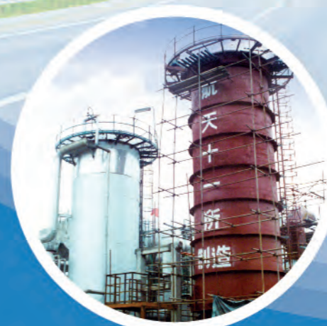
设备节能改造 Equipment Energy-saving Engineering
